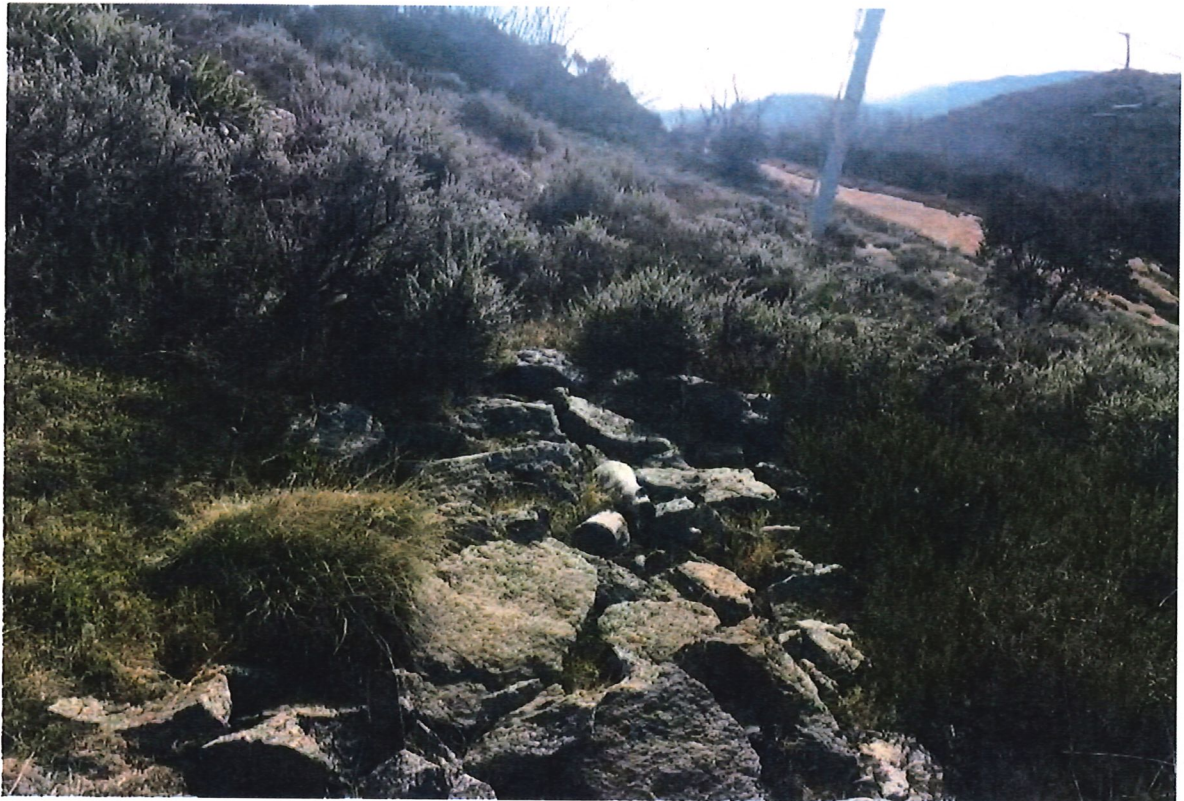
Photo 3: The new snowmaking main to the proposed Fan Gun 1 will affect some clumps of small rocks that are the result of historic slope grooming activities.
